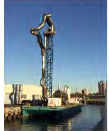
Figure III-8: AMECS Barge System
