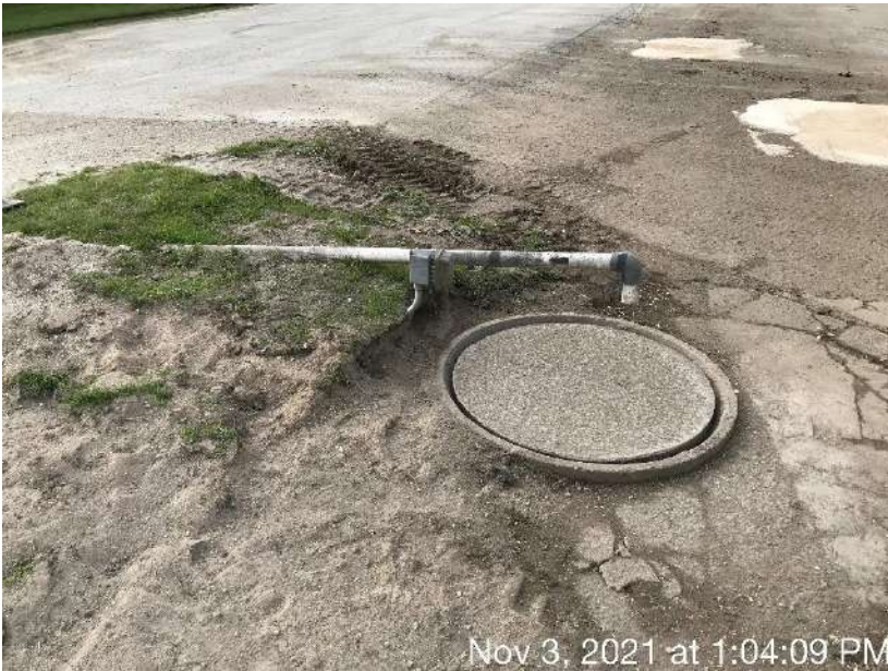
Photo 139. The second collection inlet for the northern feed storage area at Site 1. This photo was taken facing northwest. The inlet was covered to prevent stormwater collection.
