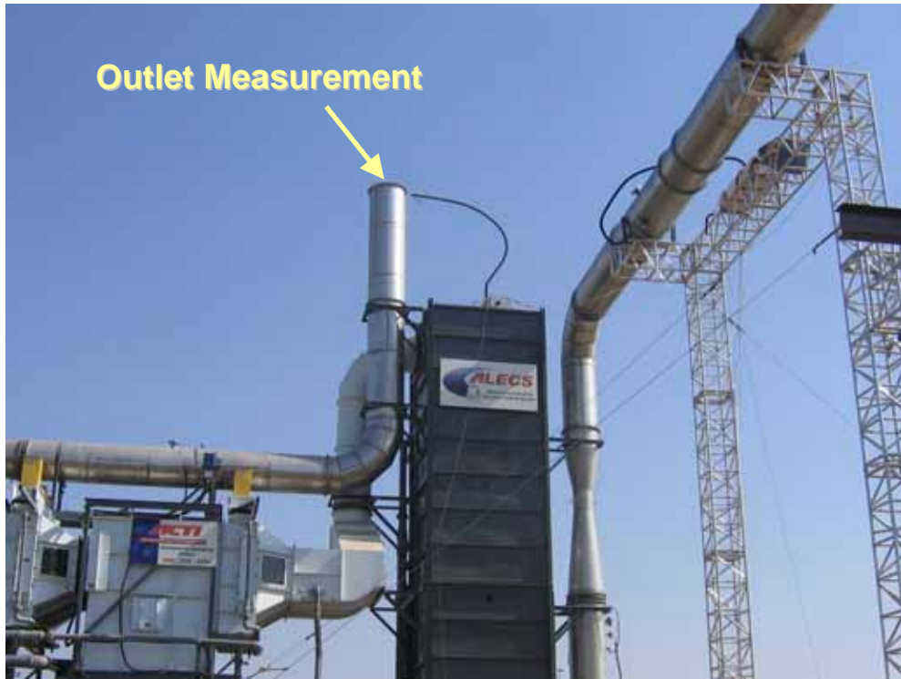
Figure 21. Exhaust Stack of the Emissions Treatment Subsystem
