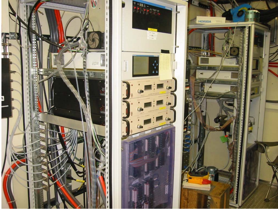
Figure 11. Continuous Emission Monitoring System
