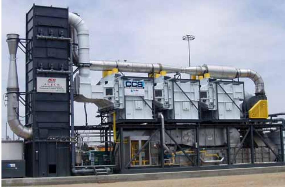
Figure 16. Emissions Treatment Subsystem in Roseville Rail Yard
