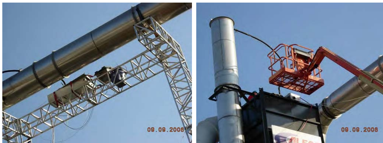
Figure 1: RAVEM installations at the ALECS inlet and outlet
