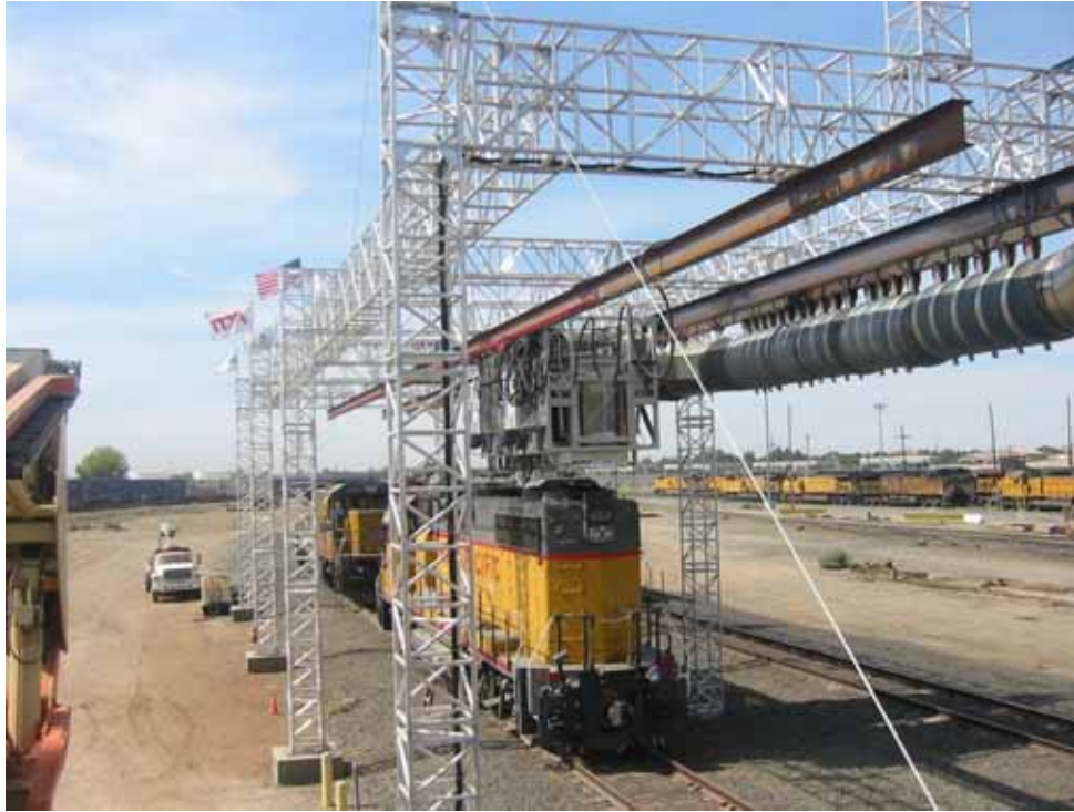
Figure 6. Overhead Structure and Intake Manifold
