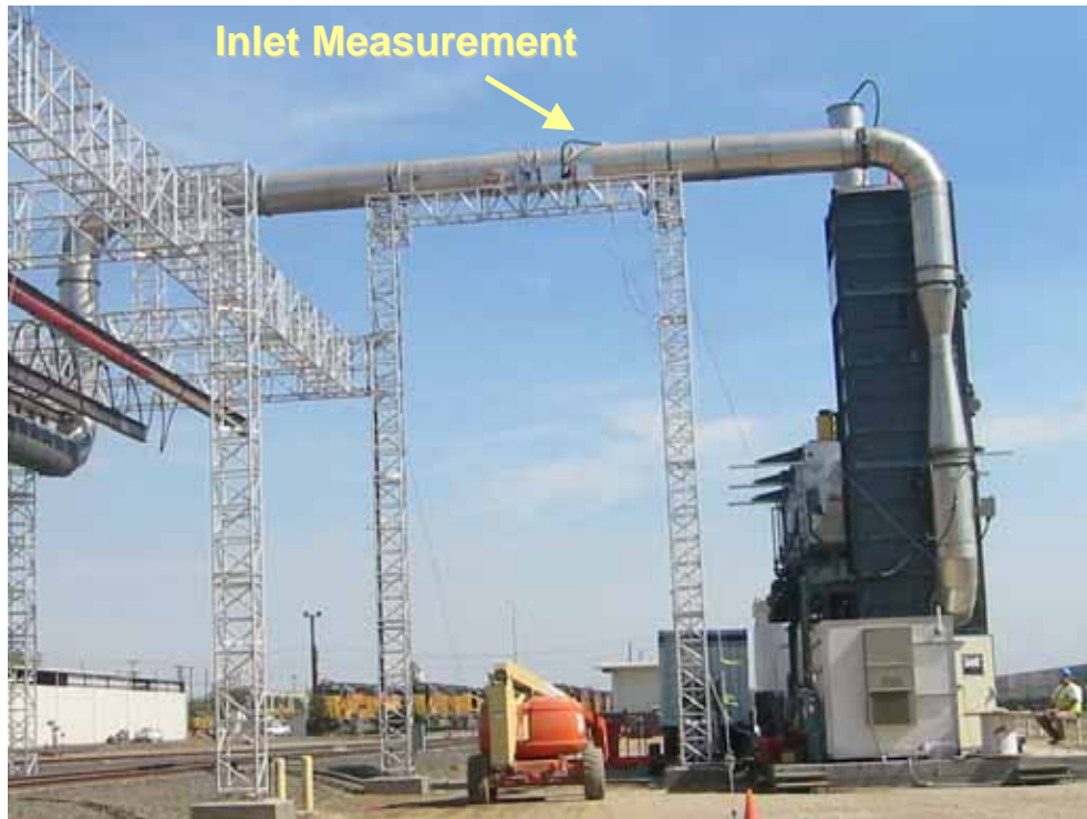
Figure 20. Ducting between the ECS and the ETS
