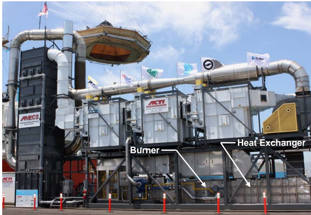
Figure 10. ETS: SCR Heat Management System
